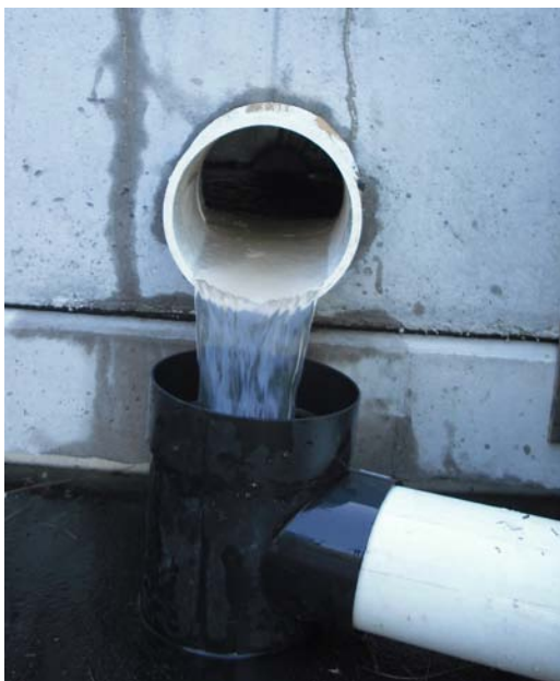
a) 6-inch outlet port from the junction box underneath the inlet
