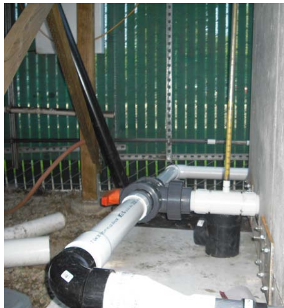
b) 3-inch outlet with 3-inch port ball valve for switching between unrestricted flow in the 3-inch pipe (background) and the 1.5-inch flow meter (foreground)
